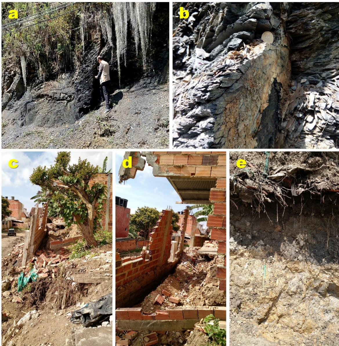
Figure 2. Occurrence of (a,b) a mudstone outcrop of the Kip3 segment of the Paja Formation along the cutting slope in the San Luis neighborhood, and (c–e) a regolith of the Kip2 segment of the Paja Formation and excavation in the Las Nieves neighborhood.
