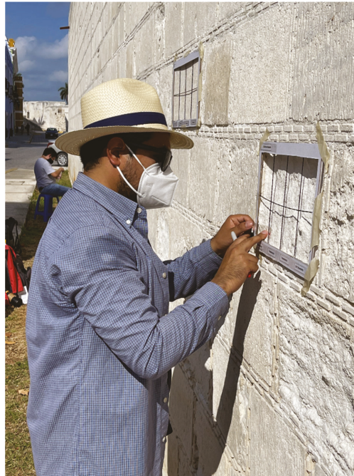
Figure 1. Limestone wall in Campeche, southern México, exhibiting a range of deterioration pathologies. Formers are being used to demarcate panels prior to treatment by spraying with carbonatogenic bacterial suspension or control solution. Replicate panels will allow statistical analysis. The aim is to increase surface hardness and reduce the detachment rate of flaking material.
