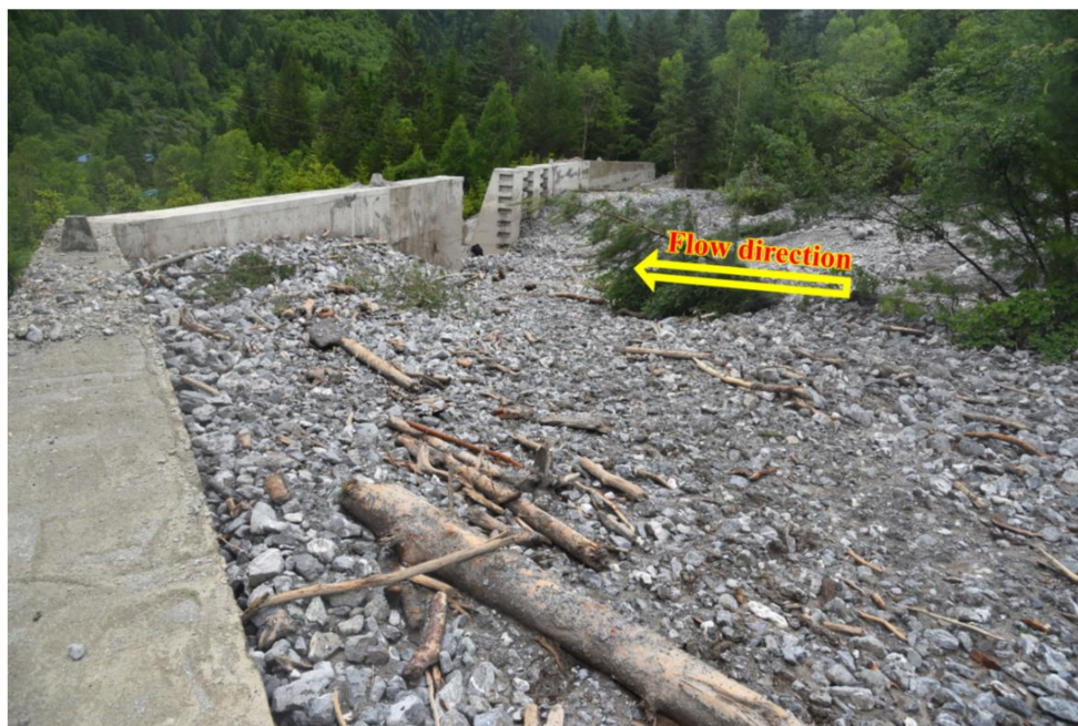
Figure 6. Overview of the reconstructed retaining wall in Zechawa Gully (taken on 23 June 2019).
