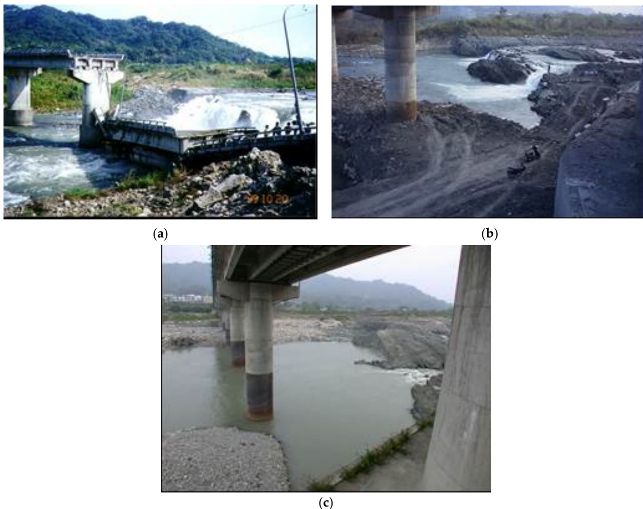
Figure 1. (a) Changed river bed and damaged bridge due to the 921 Earthquake in 1999; (b) Newly constructed bridge in the same location; (c) Water drop and local scour at the bridge piers.
