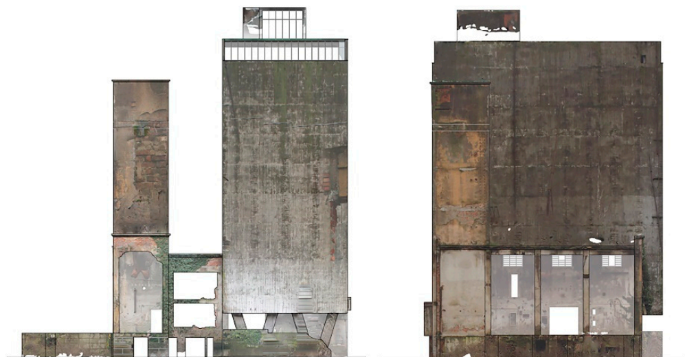
Figure 8. Image planes of two sides of the abandoned 32-m-high vegetable oil refinery building slated for demolition, obtained via close-range photogrammetry.
