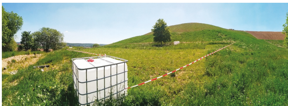
Figure 7. Preparations for the installation of the electric fence at site V2 on 19 May 2020.
