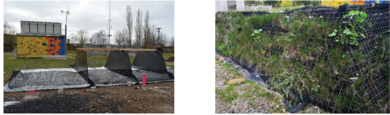
Figure 4. Left: View at the base layer of the pilot application before installation; Right: Northwest view at the greened construction in October 2020 (6 months after erection). Pictures: Schneider.
