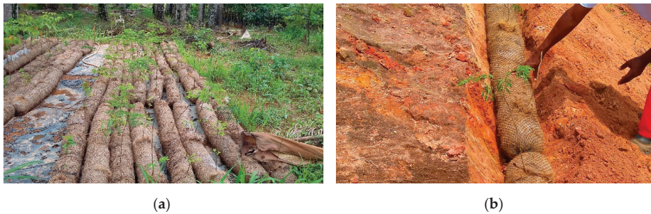
Figure A3. Organic sediment retainers associated with live elements (L-OSRs): (a) storage in the experimental units; and (b) installation of the elements in manually excavated trenches.
