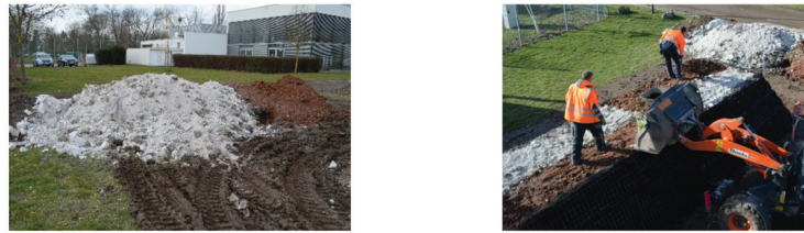
Figure 2. SBM mixed with organic soil, left: before installation, right: after installation in a pilot application. Pictures: Schneider.
