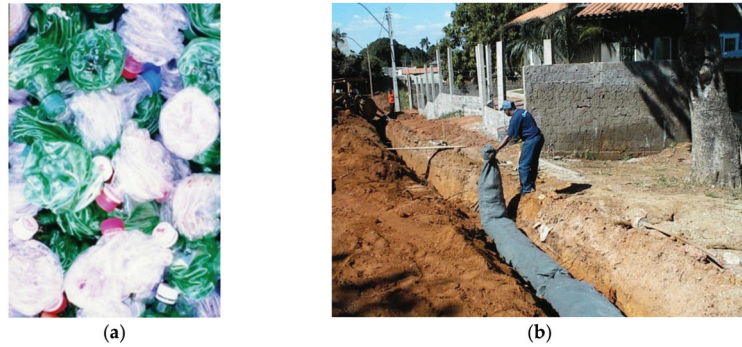
Figure 21. Alternative drainage system with a core of compressed PET bottles (images courtesy of H. Paranhos): (a) compressed PET bottles; (b) geocomposite for drainage formed by compressed PET bottles enveloped by a geotextile filter in a drainage trench.
