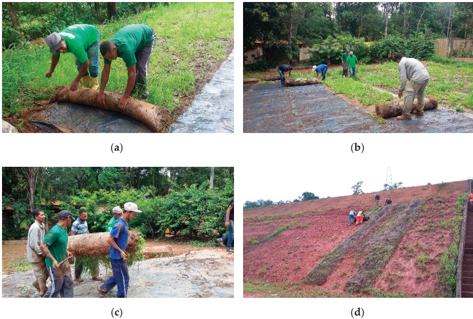
Figure A2. Live rolled erosion control products (L-RECPs): (a) cultivation at greenhouses, (b) coil-shaped collection, (c) transportation, and (d) installation of the elements in the experimental units slopes.
