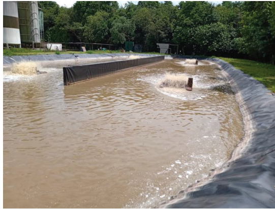
Figure 1. Sewage treatment aeration pond under operation.
