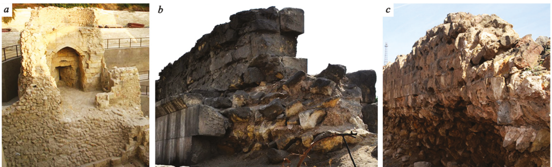
Figure 18. Examples of detachment and collapse of facing ashlar layers, exposing the inner core layer built of rubble stone masonry: (a) Bab al-Mahruq , (b) Bab Qaytbay , and (c) northeastern historic Cairo wall.
