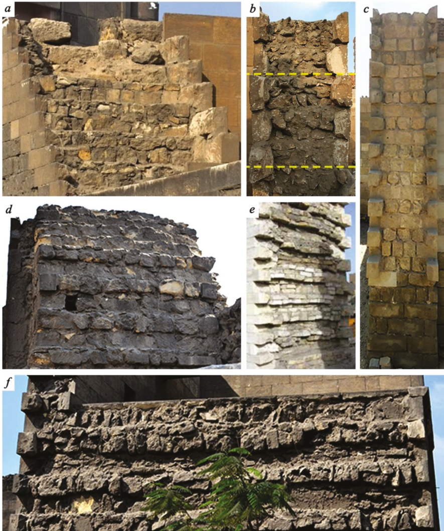
Figure 16. Different cross-sections of multiple-leaf stone masonry walls with the internal leaf built by successive layering of rubble stones and mortar bedding with horizontal courses: (a) Complex of Al-Sultan Hasan , (b) Complex of Sultan al-Ashraf Barsbay , (c) Qubba al-Amir Tarabay al-Sharifi , (d) and (f) perimeter wall of Bab Qaytbay ; and (e) the aqueduct ( Majra Al-Uyun ).
