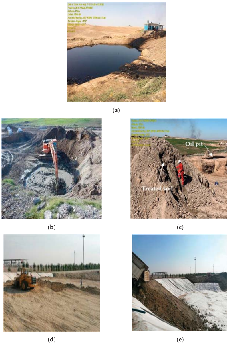
Figure 3. The treatment process of pollutant soil: (a) the oil pit before treatment; (b,c) the treatment of contaminated soil in the oil pit; (d) reconstruction and lining of the oil pit; and (e) backfilling of the pit with treated soil and leveling.
