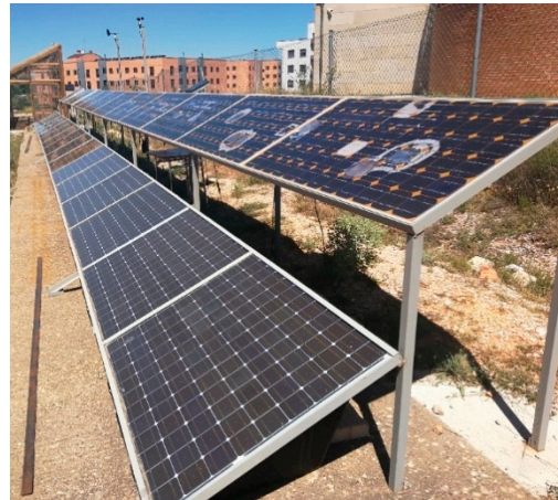
Figure 6. Photovoltaic (PV) installation in Campus Duques de Soria.
