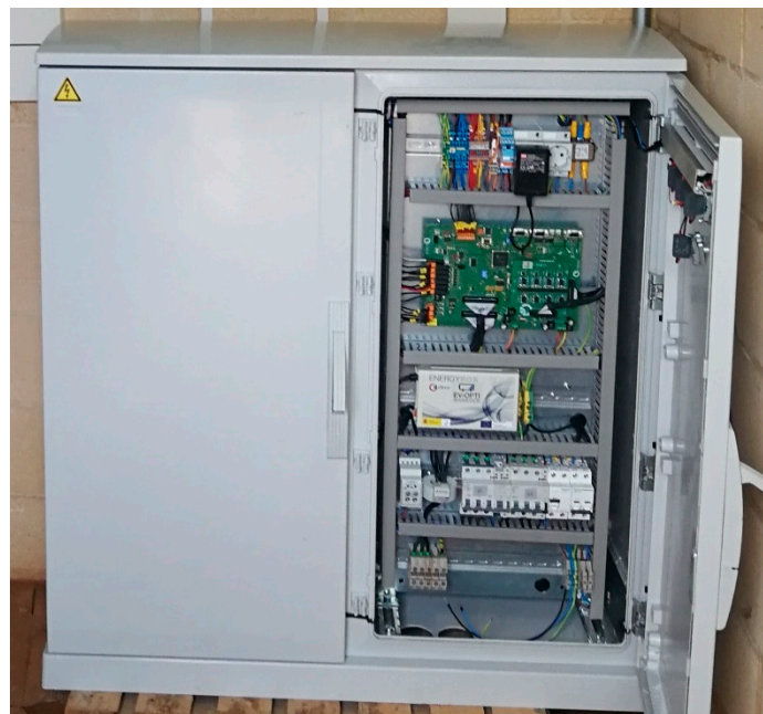
Figure 4. Bidirectional power inverter of the Campus Duques de Soria of the University of Valladolid.
