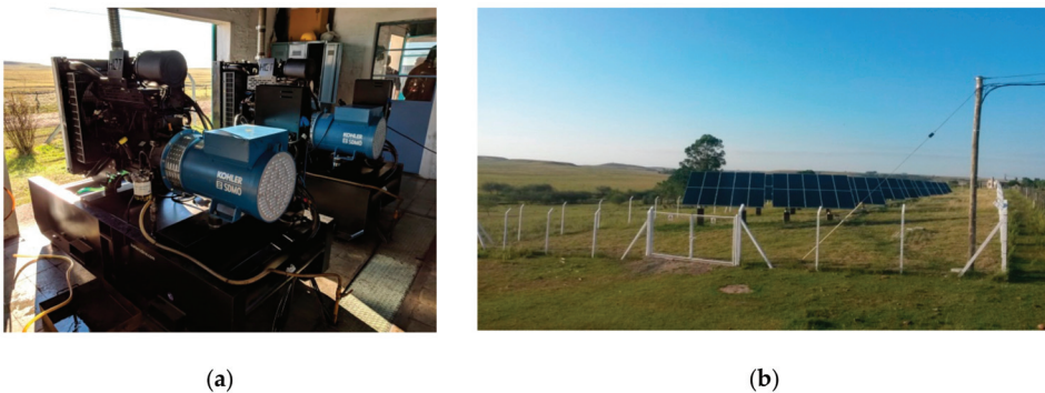
Figure A2. (a) The inside of the gensets building with the two diesel generators; (b) A general view of the solar PV generator.
