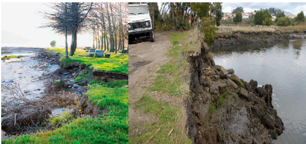
Figure 2. Cardielos (left panel) and Portuzelo (right panel) sections in 2010, previous to the bank reinforcement, where an apparent bank collapse is visible.
