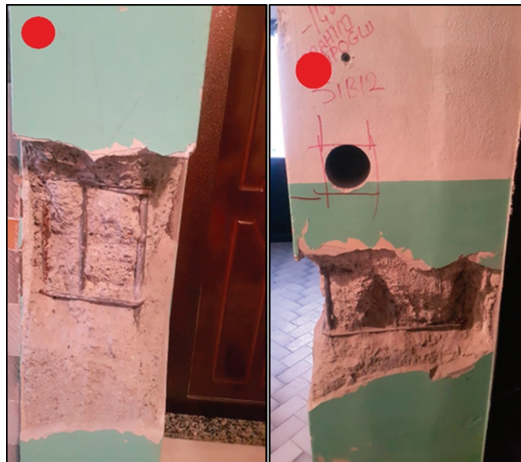
Figure 5. Column damages of a building to be demolished. Photos were provided by the study participant upon request of the authors. The intensity value provided by the participant was “Strong”.
