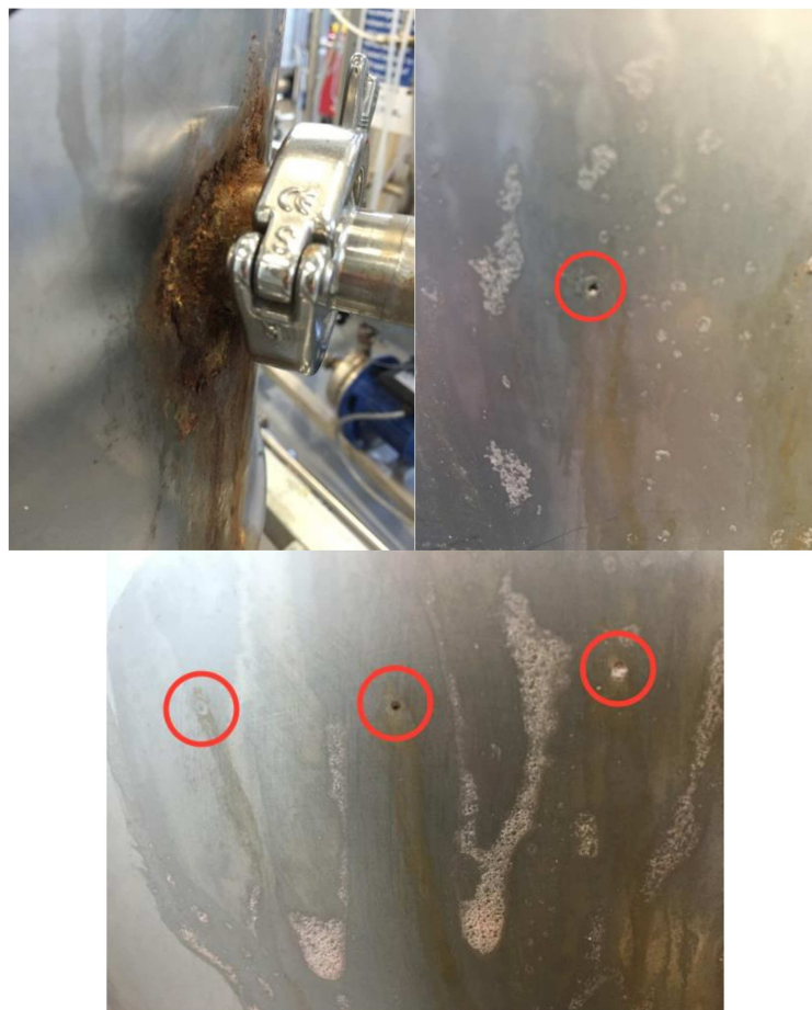
Figure 9. Swanssea feed tank corrosion. Top left, rusting around the tri-clamp connection. Top right and bottom, pitting on the vessel surface.
