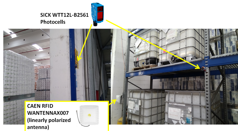
Figure 7. Photocells installed at one of the UHF-RFID Smart Gates.
