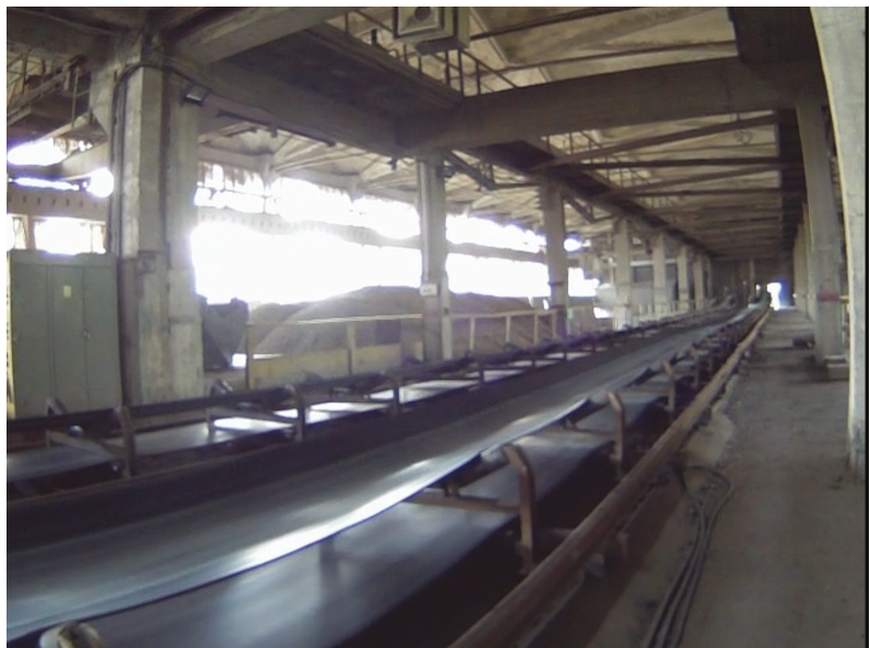
Figure 1. A general view of the belt conveyor.
