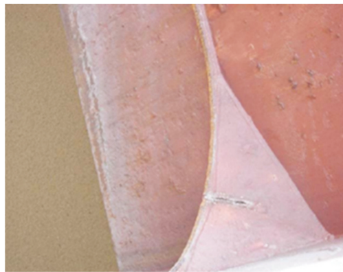
Figure 1. A fatigue crack in the hatch corner of a certain ship.
