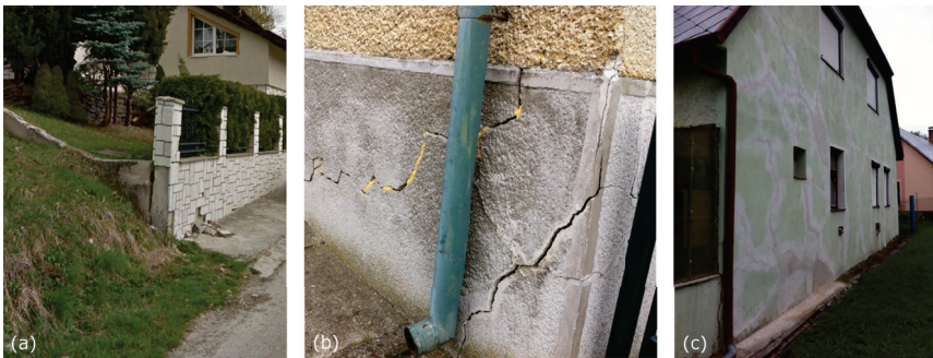
Figure 3. Photo-examples of structural damage in Hradec and Velka Lehotka (case study 1) caused by local slope deformations, (a) April 2012, Photo courtesy: Google Street View; (b) and (c) July 2017.
