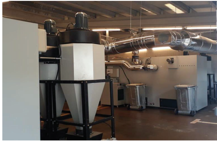
Figure 8. Thermal system in the Pontevedra campus of the University of Vigo.
