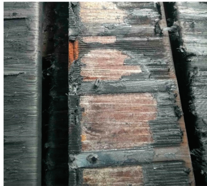
Figure 1. Electrical Erosion (2012)—Stator Bars.
