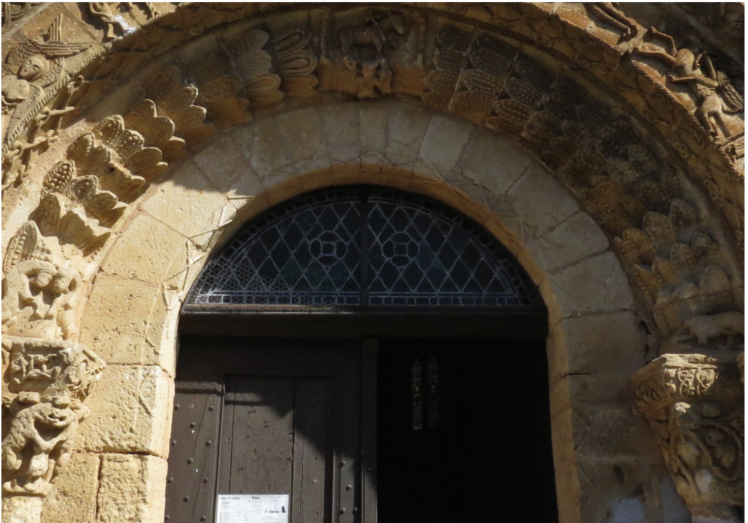
Figure 10. Palm-tree ribbons and door frame, detail of archivolt, west façade, Saint-Martin Church , 12th c., Besse, Dordogne, Nouvelle-Aquitaine, France. ©Author.
