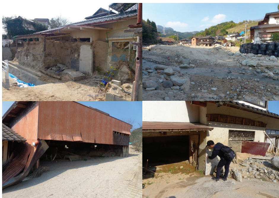
Figure 3. Situations of the flood disaster in the Shirakitani River Basin (as of March 25, 2018).
