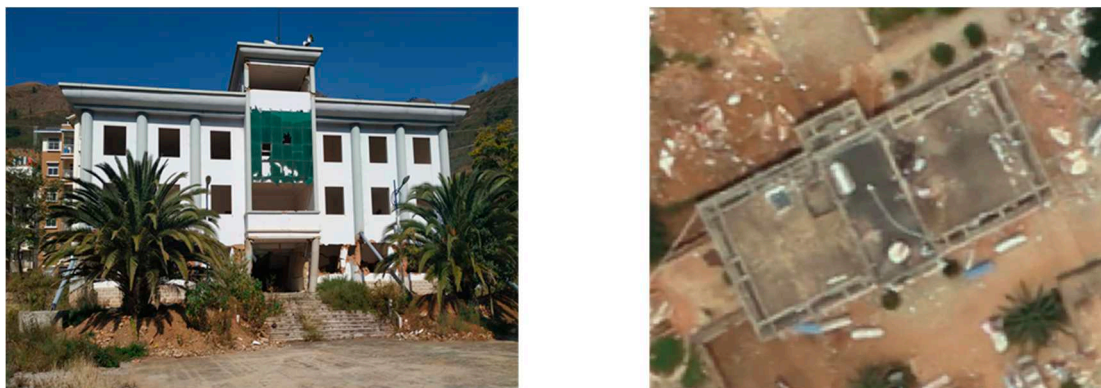
Figure 6. Example of underestimated building damage by visual interpretation of an aerial image. Left: ground photo; Right: aerial image. The collapse of the building is not visible on the aerial image.
