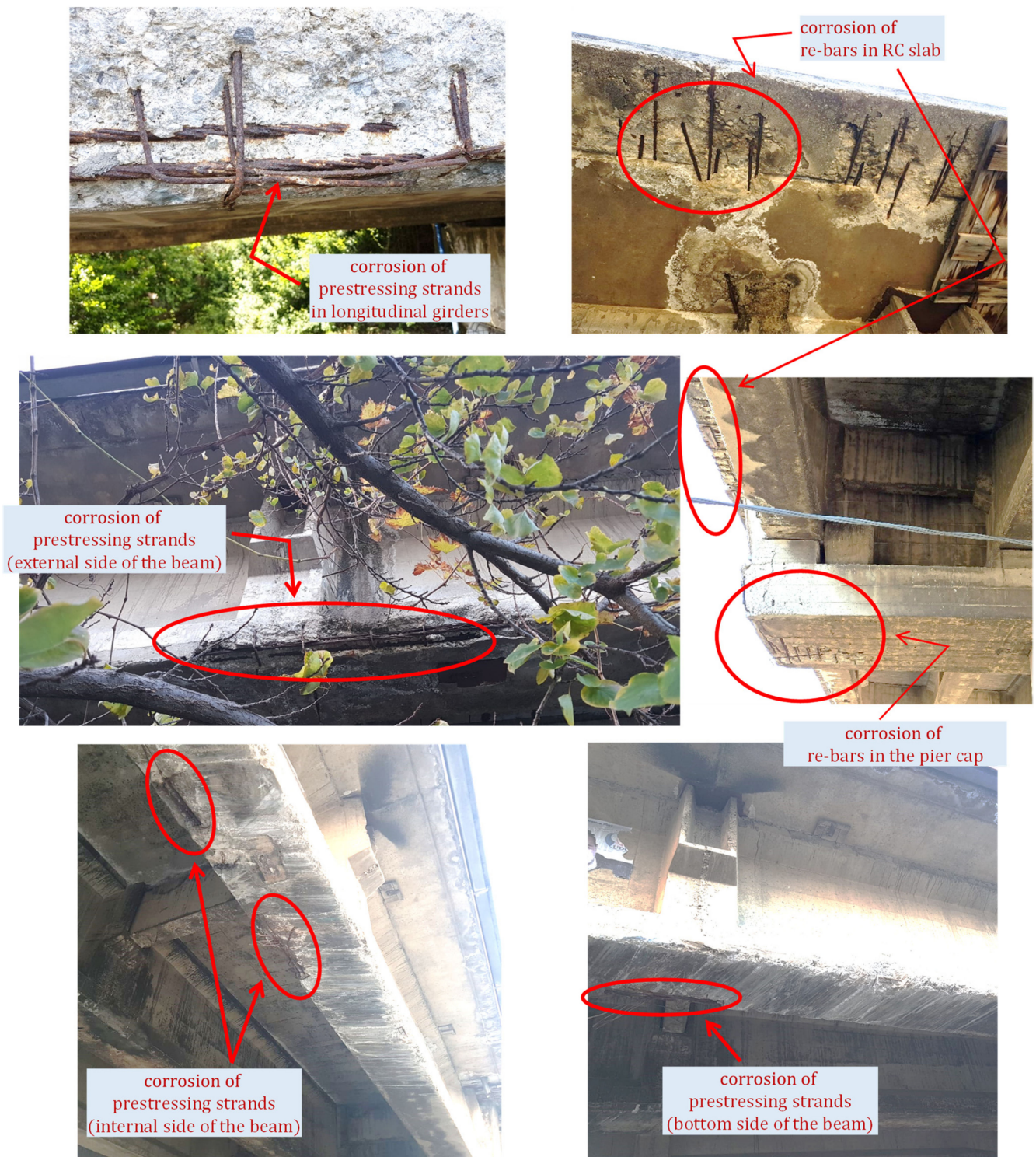
Figure 3. Widespread corrosion state of the Longano viaduct detected from visual inspection.
