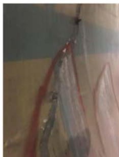
Figure 2. Cracking of the tunnel lining.
