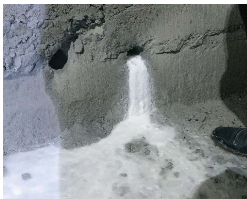
Figure 1. Crystallization and clogging in drainage pipes in the Baoligang Tunnel of the Emeishan-Hanyuan Expressway.
