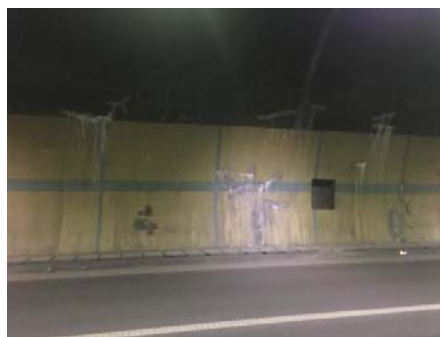
Figure 2. Cracking and leakage of the tunnel lining.
