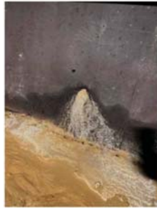
Figure 3. Tunnel drainage pipe blockage by crystals.
