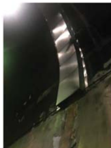
Figure 1. Water receiver at lining leakage.
