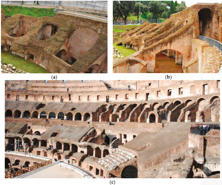
Figure 7. Examples of the structure built as a support of the podium with a double purpose, upholding the structure of the seats and corridor for the public to reach their seats: (a,b) Circus Maximus in Rome; (c) Flavius Amphitheatre (Colosseum) in Rome.
