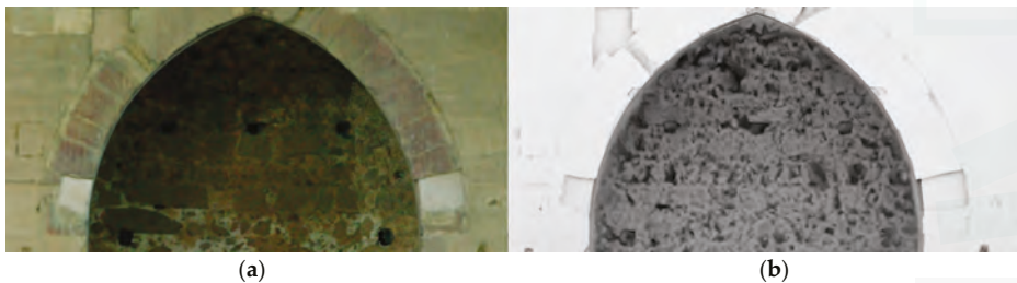
Figure 10. Efflorescence in the stone: (a) the RGB image showing a smooth surface; and (b) deterioration of the stone by alveolization of the materials shown by ambient occlusion.
