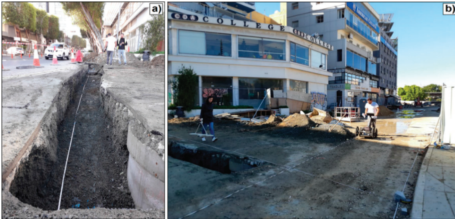
Figure 12. Corner between Evagorou Avenue and Omirou Avenue: the excavated trench (a), GPR and EMI data acquisition (b).
