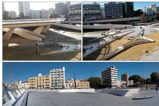
Figure 4. Eleftheria Square project: photographs of the work in progress captured in December 2019.
