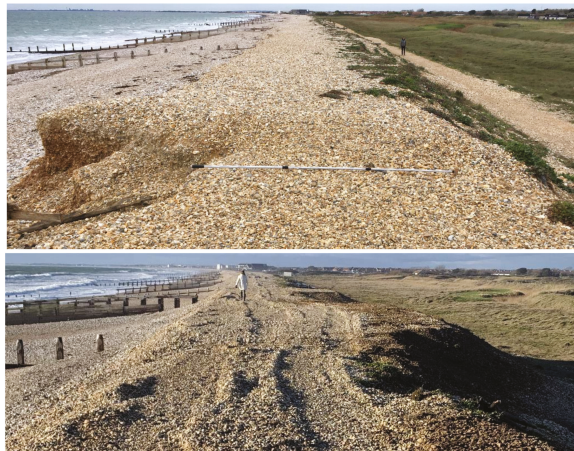
Figure 21. Management intervention in 2021 showing before (top on 12 October 2020) and after (bottom on 29 January 2021) groyne plank removal and increasing the CSA behind the groyne at the back of the beach. Pole in the top photo is 3 m long.
