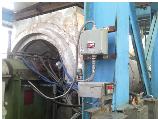
Figure 6. The local-data acquisition system.
