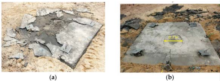
Figure 11. Damage of the multi-layer pavement after blast loading: (a) damage pattern of the AC layer in field blast test; (b) damage pattern of the HSC layer in field blast test.
