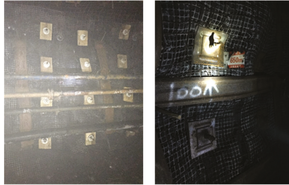
Figure 21. The actual state of displacement of surrounding rock in tail entry 3105.
