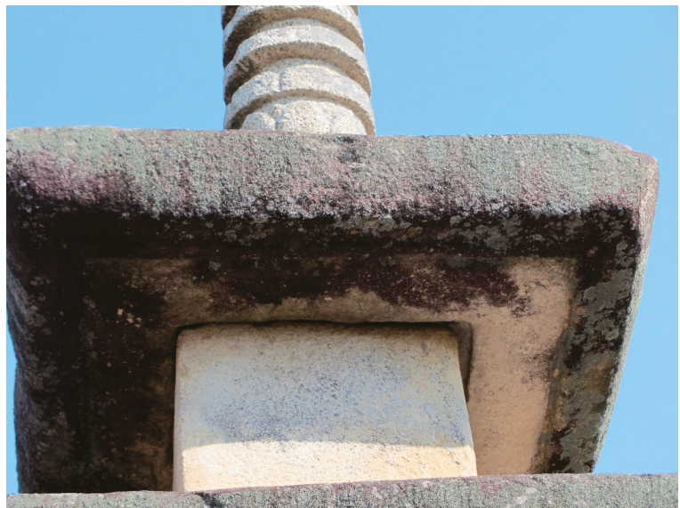
Figure 2. The groove below the eaves at the top story of the Ishidōji pagoda.
