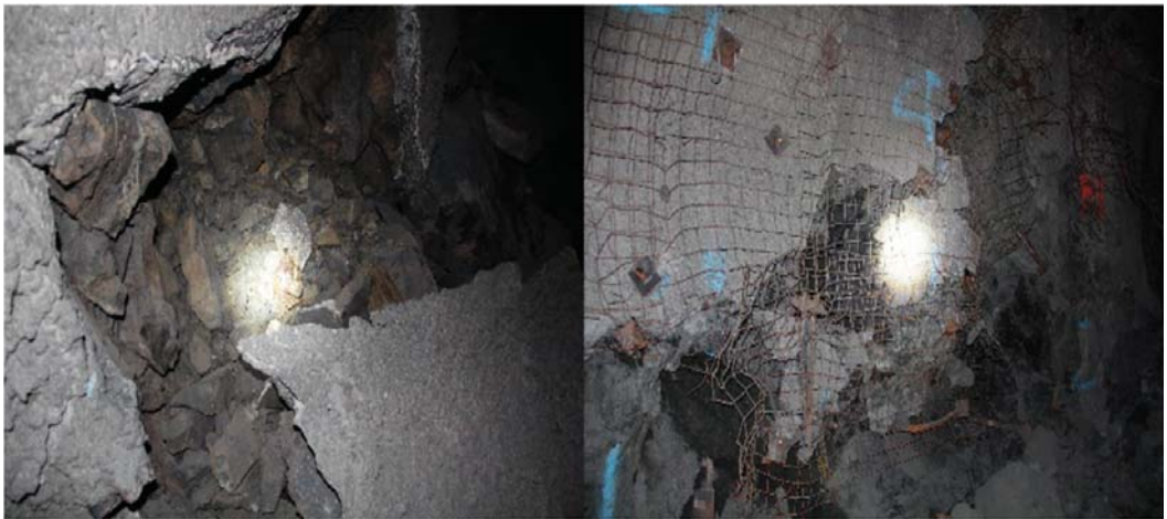
Figure 10. Failure cases near the stope access.
