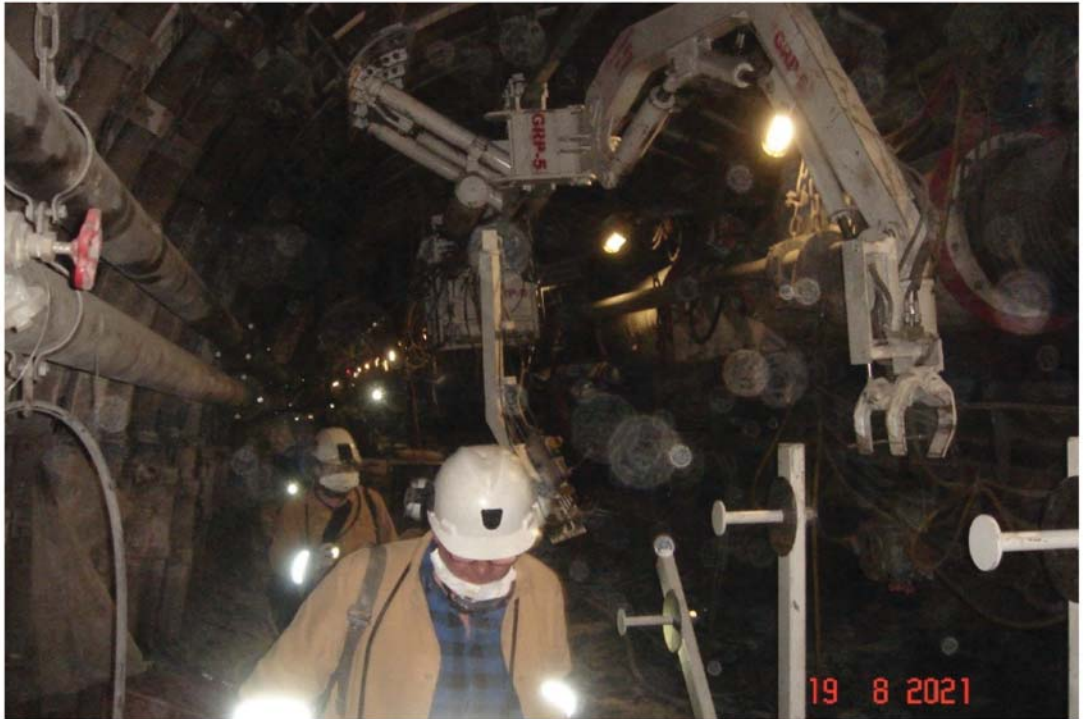
Figure 20. View of the MZZ-M installed in an underground excavation.
