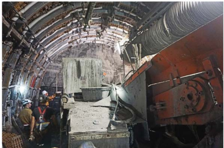
Figure 2. View of the mining face of a gallery drilled with a roadheader.
