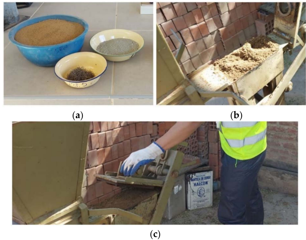
Figure 4. Preparation of soil–cement blocks: (a) preparation of materials, (b) placement of mixture, and (c) compaction.
