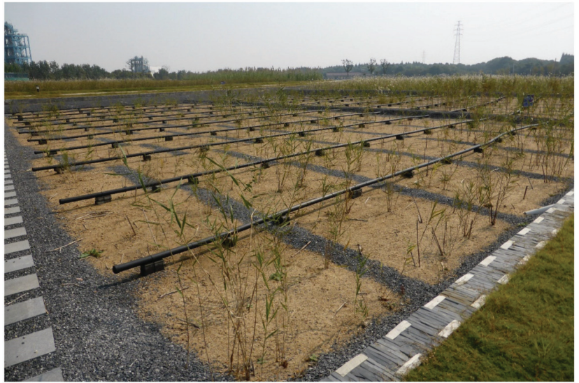
Figure 11. Wastewater distribution pipes at Changshu Advanced Materials Industrial Park VF CW, Suzhou, Jiangsu Province, PR China. Photo Jan Vymazal.
