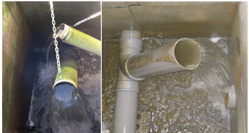
Figure 10. Water level maintenance. Left: outflow pipes hanging on a chain at CW Waikeria, New Zealand. Right: swiveling elbow at CW Bouvron, France. Photo Jan Vymazal.
