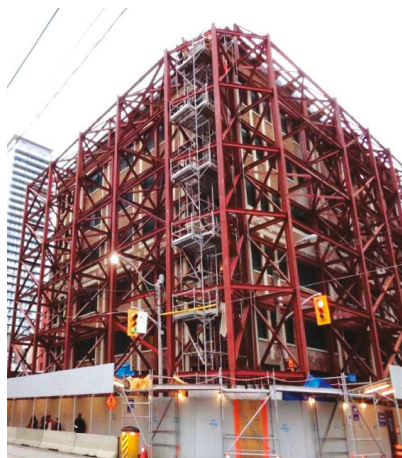
Figure 12. Temporary protection for the façade wall in the form of a steel frame structure [1].
