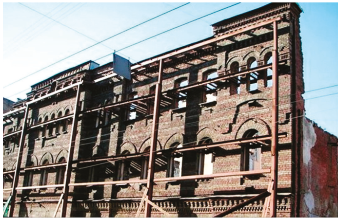
Figure 14. Temporary protection for a façade wall in the form of a steel buttresses (photograph by authors).
