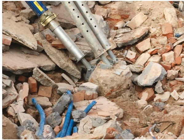
Figure 17. Anchoring of the PERI Push-Pull Props system to the pile head (photograph by authors).
