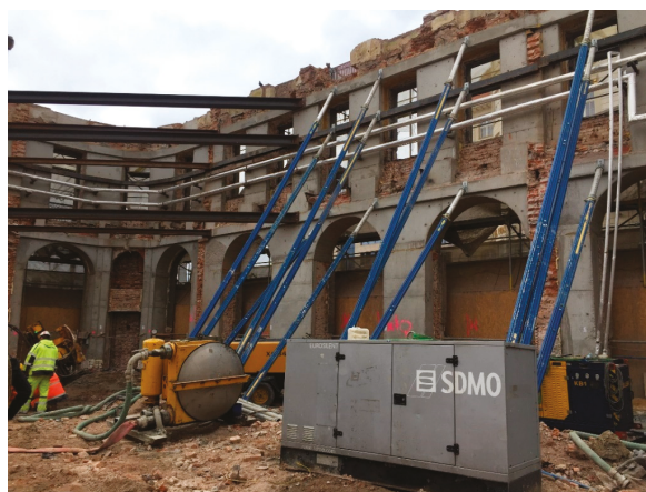
Figure 16. Supporting the walls of the existing building in 3 levels with the PERI Push-Pull Props system (photograph by authors).
