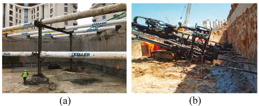
Figure 2. Structural solutions to ensure the stability of a deep excavation: (a) bracing struts, (b) ground anchors (developed by authors).
