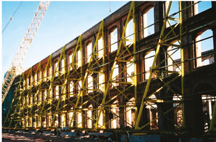
Figure 11. Temporary protection for the façade wall in the form of a strut-and-tie steel structure [3].
