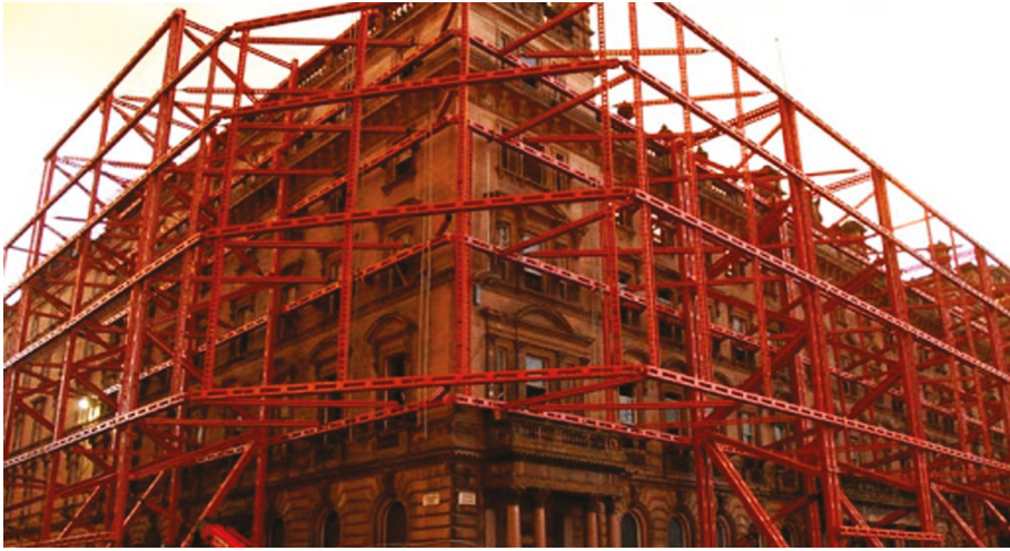
Figure 13. Temporary protection for a façade wall in the form of a steel frame structure [22].
