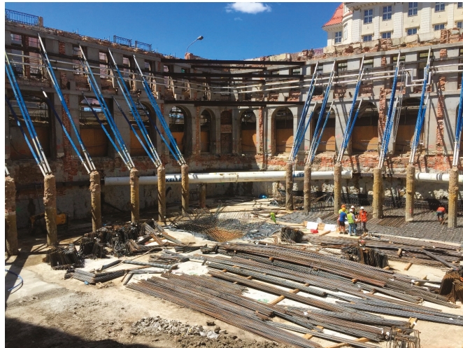
Figure 15. Temporary protection for a façade wall made of the PERI Push-Pull Props support structure (photograph by authors).
