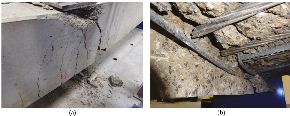
Figure 10. Failure of NSC beam: crack pattern (a), and rupture of pretensioned reinforcement (b).
