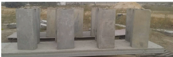
Figure 2. Concrete blocks setup in the coastal zone, with the proper bracing on top and isolation from sand.
