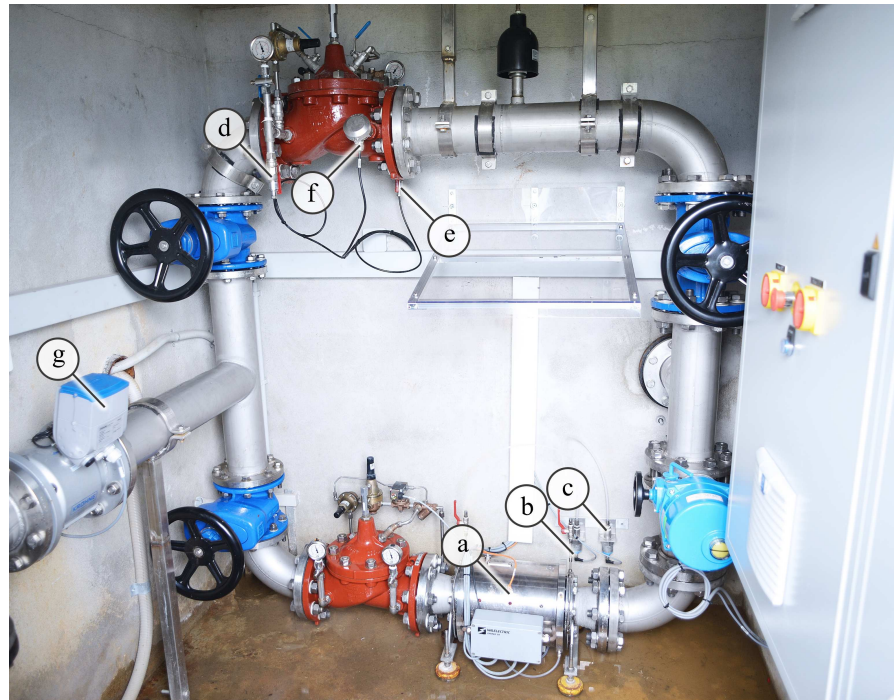
Figure 11. Installed DuoTurbo pilot in a drinking water supply network at Savièse (VS Switzerland). The positions (a–g) refer to the instrumentation list given in Table 7.
