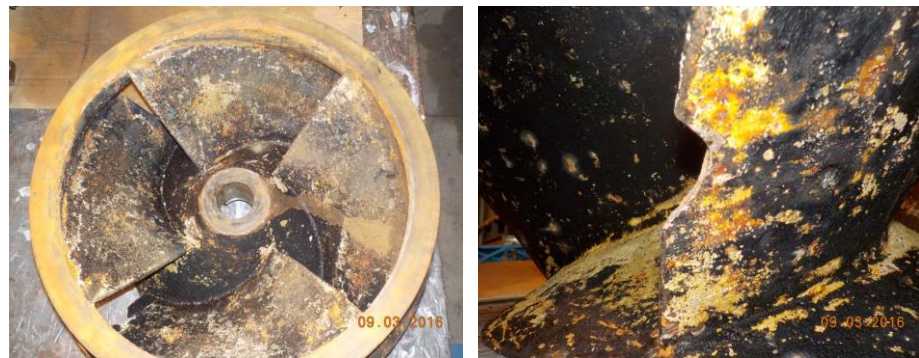
Figure 16. Impeller failure of the pumping unit no. 3 on 9 March 2016.
