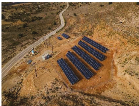
Figure 16. Photo of the Tilos HPS PV plant, installed at the central part of the island.
