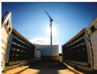
Figure 17. Photo of the Tilos HPS BESS, installed at the northwestern part of the island.
