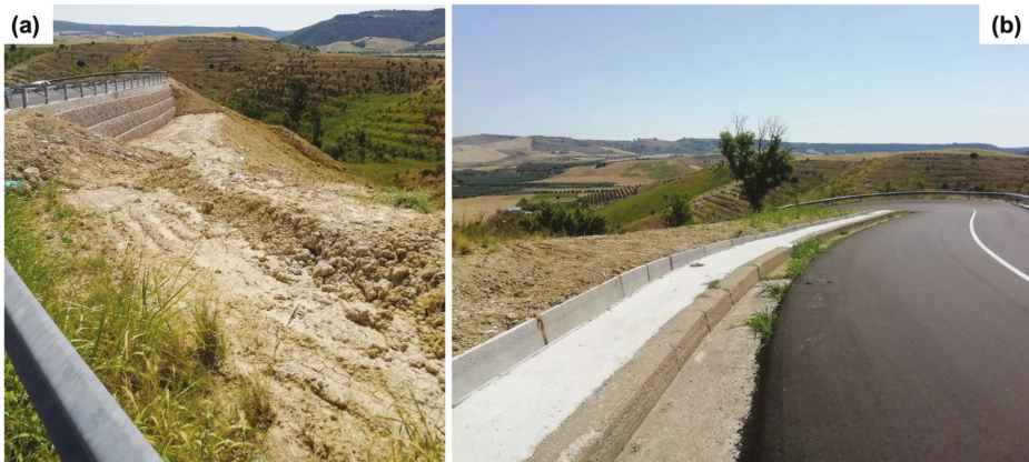
Figure 12. Pictures of the road section in Montescaglioso village corresponding to the area where target P1 in Figure 6 is located.
