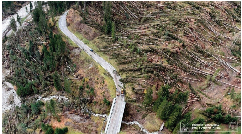
Figure 7. Aerial view of one of the areas hit by Vaia in Friuli Venezia Giulia [2].
