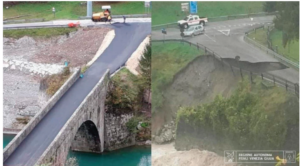
Figure 2. Aerial view of one of the areas hit by Vaia in Friuli Venezia Giulia [2].
