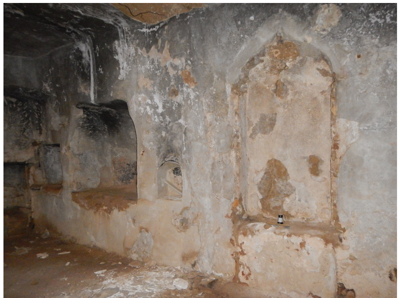
Figure 4. View of the east wall, St. Mary of the Cave, Famagusta (Photo: Andreas Foulías).
