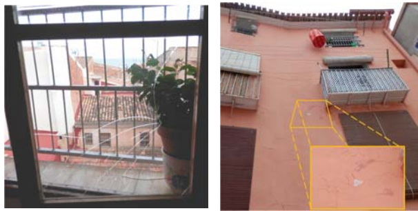
Figure 25. Some damages detected after tests.
