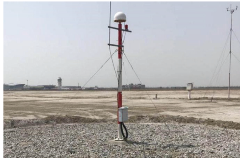
Figure 10. BDS GBAS antenna mounted on the ground near the runway at the Dongying Airport in Shandong, China.
