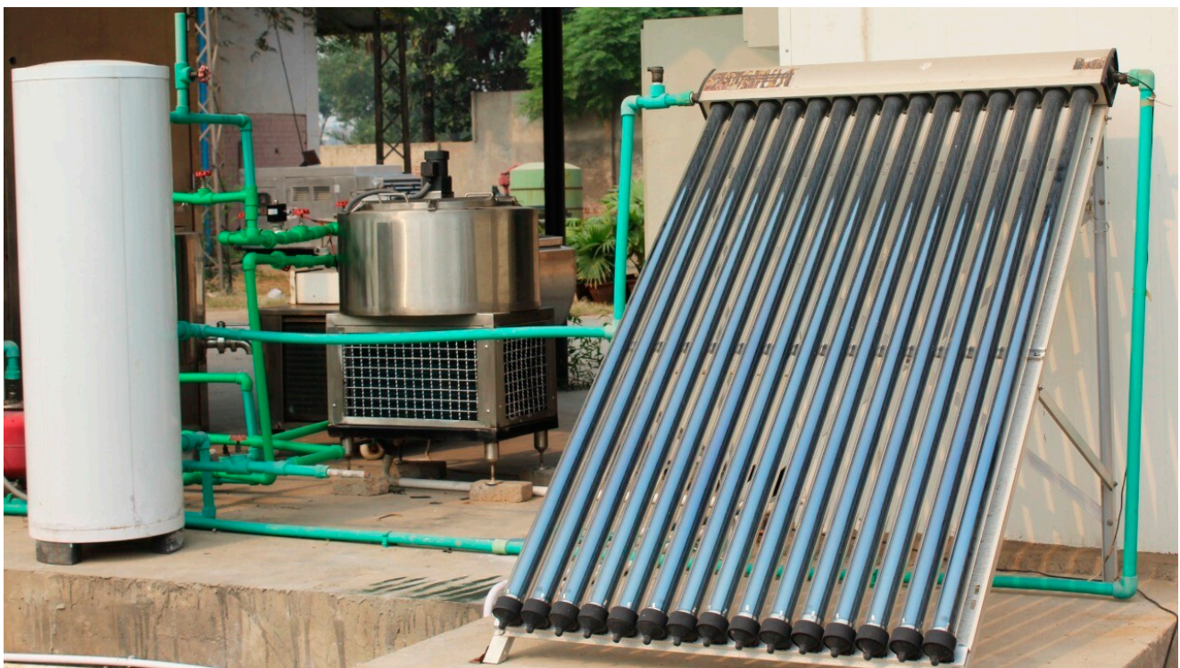
Figure 3. Pictorial view of the installed solar-assisted yogurt processing unit.
