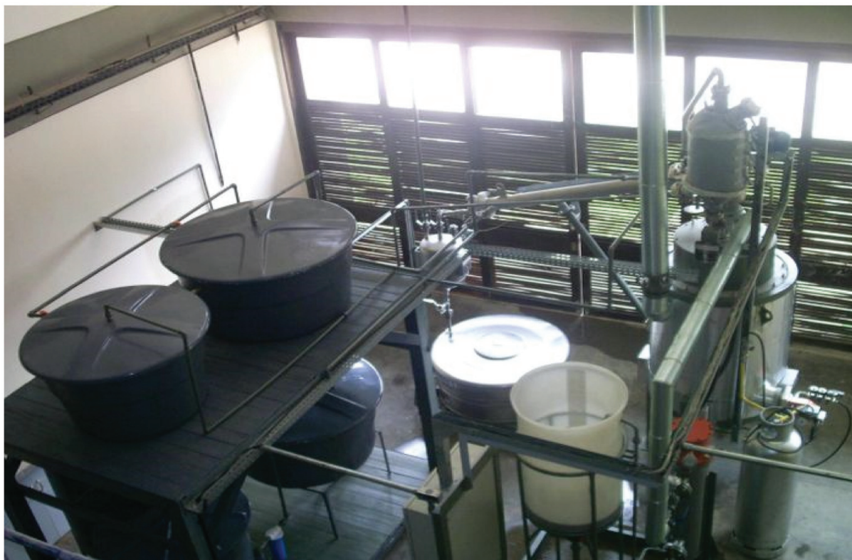
Figure 5. View of the pyrolysis unit in pilot scale.
