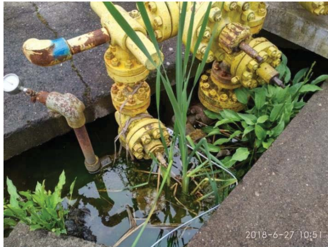
Figure 9. Example of the unsatisfactory condition of a gas well at its mouth, (source: elaborated by authors).
