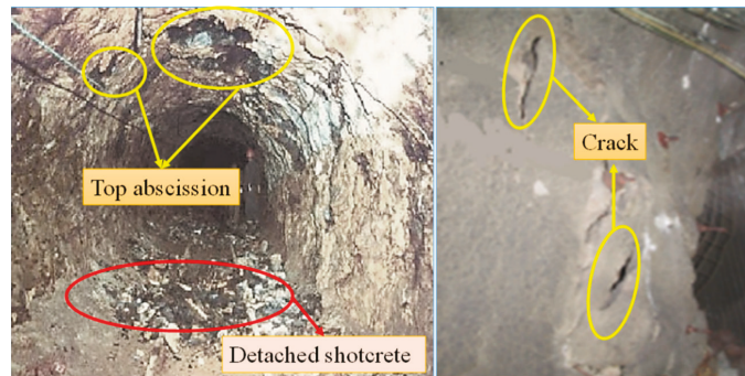
Figure 3. Shotcrete layer falling off at high temperature.
