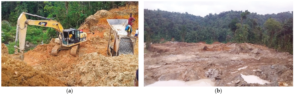
Figure 4. Invasion by illegal miners. (a) Machinery used for gold extraction; (b) deforestation of the affected area.
