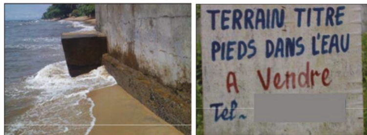
Figure 24. Land pressure on the coast in Kribi. The photo on the left shows the foundation of a private hotel in Kribi, directly built on the coastline (titled land—feet in the water—for sale). The photo on the right was taken -10 m from the shoreline. Indeed, since the entry into office of the PAK, there has been a major land race in this city, which has become the new growth pole of Cameroon. Land sales are multiplying, even in the private domain of the state, and advertisements are multiplying on the internet. The 2008 state law prohibiting the occupation of land 50 m from the coastline has thus been flouted.
