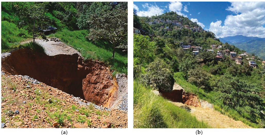
Figure 3. Sinkhole in the province of El Oro, city of Zaruma. (a) Sinkhole formation; (b) houses at risk due to sinkhole formation.
