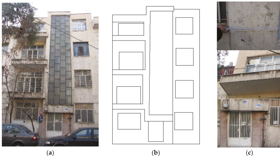
Figure 2. Illustrative example of one case study analysed in Tehran: (a) photograph of the façade; (b) diagrammatic sketch to represent the anomalies observed; (c) direct measurements and identification of different anomalies in the natural stone cladding.
