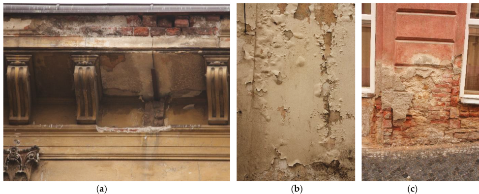
Figure 9. Examples of non-structural failures caused by the effects of the external environment, especially the synergic effect of increased moisture levels and temperature, which are accompanied by chemical, mineralogical and biological processes in structures from the second half of 19th century and the start of 20th century: (a) damage of the ledge and its surface finishes, visible salt efflorescence; (b) closed and open blisters in the surface layers due to their low diffusion permeability; (c) extensive damage to the plinth part caused by the long-term effect of humidity and salts.
