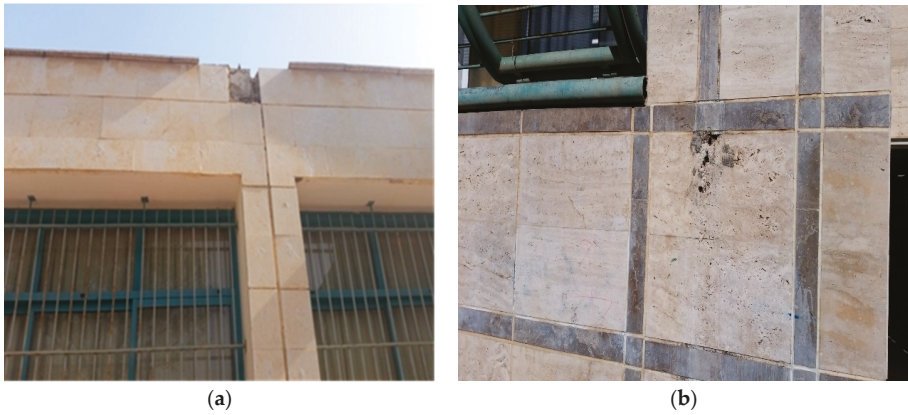
Figure 6. (a) Deteriorated exterior stone cladding. (b) Cracked stone claddings.
