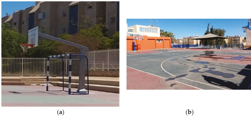
Figure 5. Sports—(a) unprotected basket column and (b) poorly maintained basketball surface.
