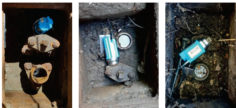
Figure 2. HWM PermaNET SU loggers deployed on hydrant control valves in different locations.
